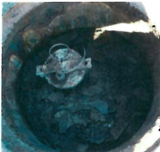
ATG Probe (unleaded) – wires are intact
