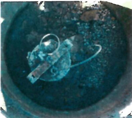
ATG Probe (plus) – wires are intact
