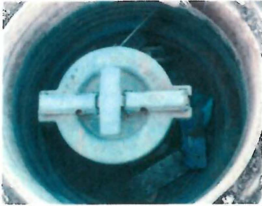
Spill bucket (unleaded) – Old tags and debris in spill bucket.
