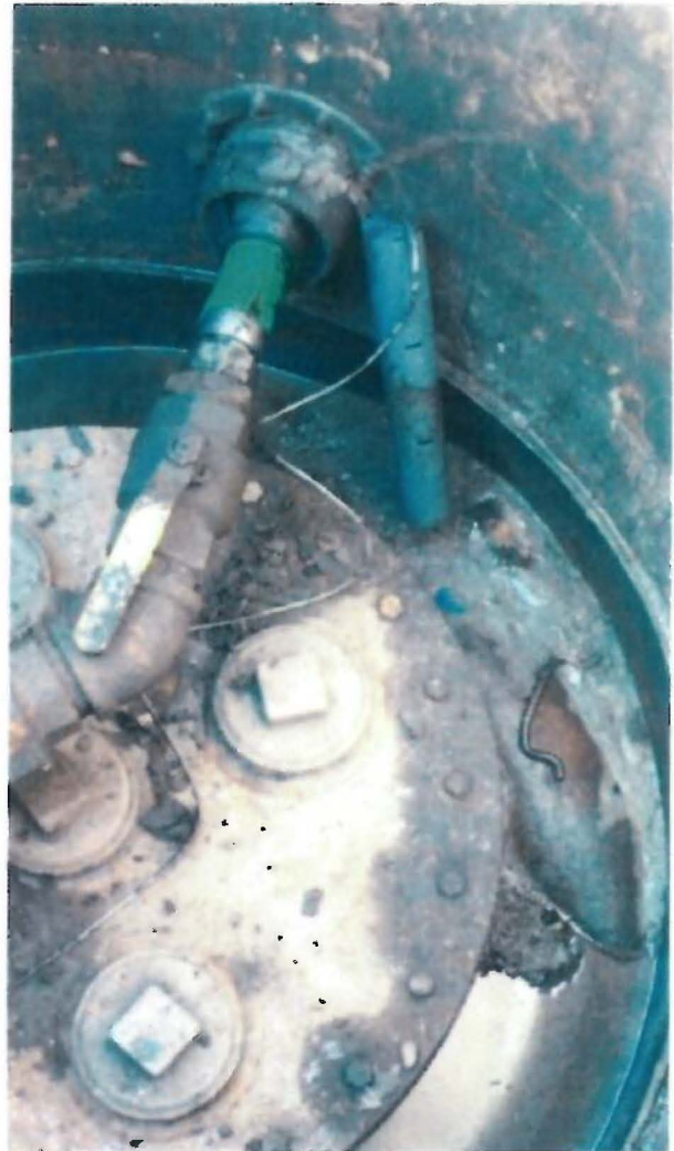
Sump shows dirt and debris
