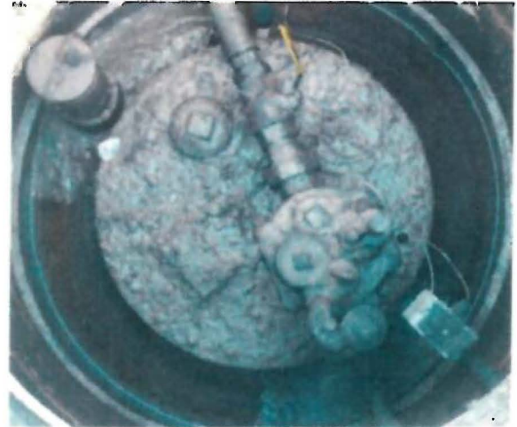
Sump (diesel) – Dirt & debris in sump; access to interstitial sensor for Tank 3 is in upper left of photo (but Tank 3's interstitial sensors in ATG machine's liquid status)
