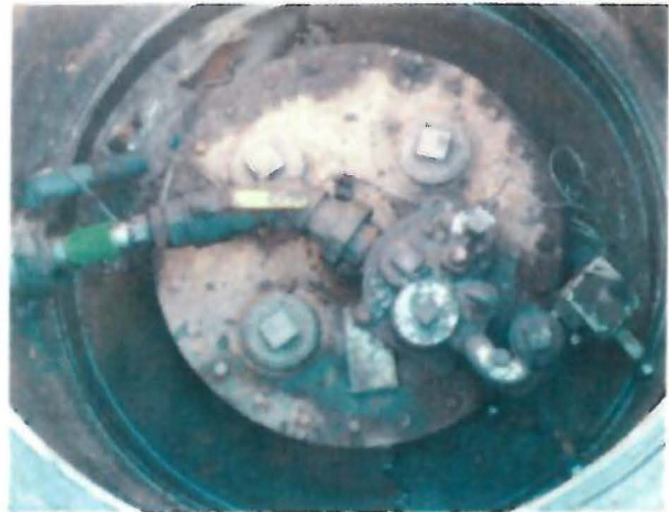
Sump (premium) – Dirt & debris in sump;
