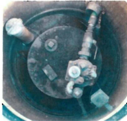
Sump (plus) – Dirt & debris in sump; access to interstitial sensor for Tank 2 is in upper left of photo
