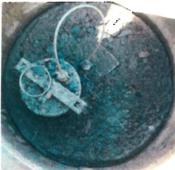
ATG Probe (diesel) – wires are intact
