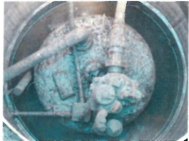
Sump (diesel) – Dirt & debris in sump;
