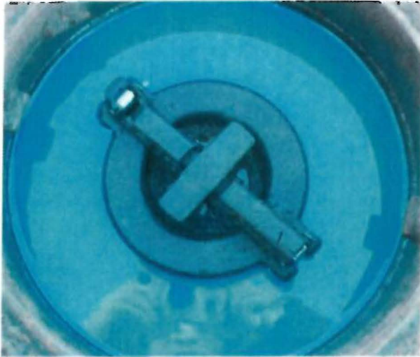
Spill bucket (diesel) –Intact, product found in spill bucket. Product in spill bucket was too full to open fill cap.
