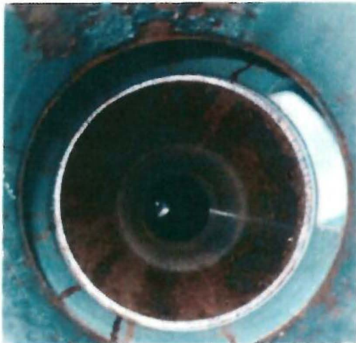
Fill port (unleaded) – records indicate ball floats for overfill protection
