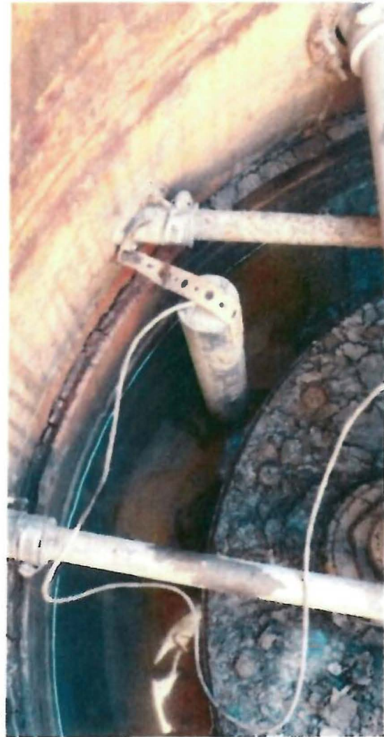
Sump sensor placed higher up in sump.
