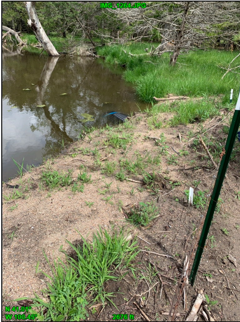
Photo shows culvert connecting the Platte River to the new excavated channel to the south.
