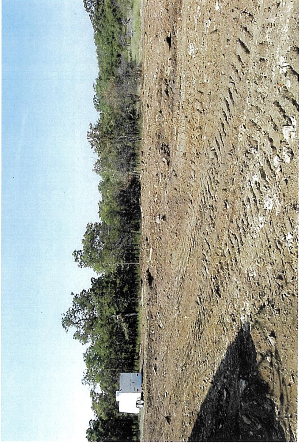
Photo 2 taken southwest. Old pit locations were present here before being filled with dirt.
