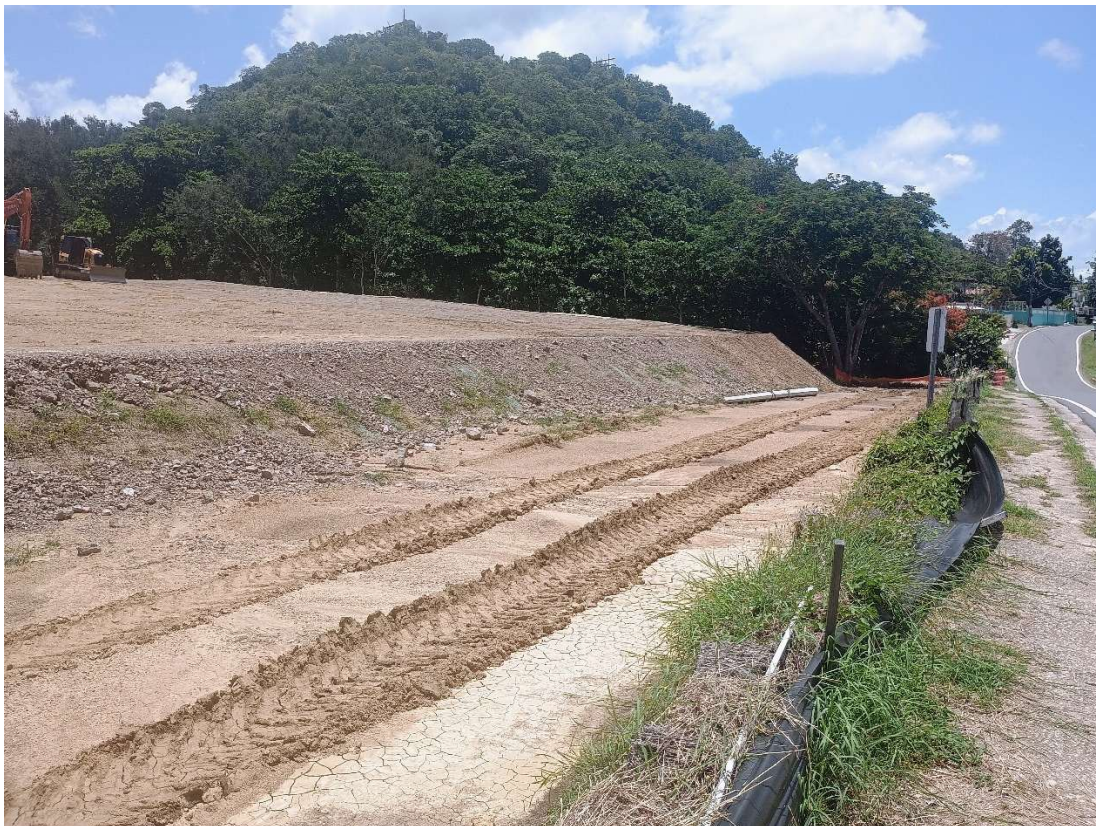
Retention basin located at the south perimeter adjacent to PR 413-Road Silt fence needs to be fixed but hay bales and a grass buffer established prior to the silt fence.
