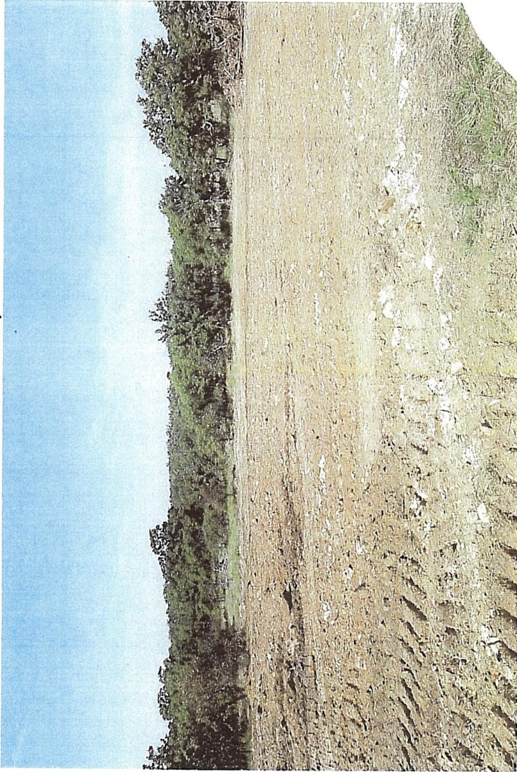
Photo 3 taken west. Location cleared for drilling. Some wet spots were pits were filled in.
