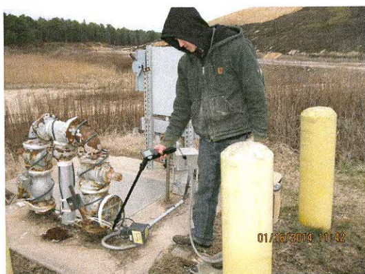
Exhibit 21 - Cell 3 Secondary Pump Station 1-16-14
