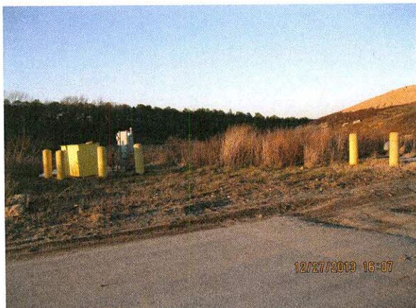
Exhibit 9 - Cell 3 Secondary Pump Station 12-27-13
