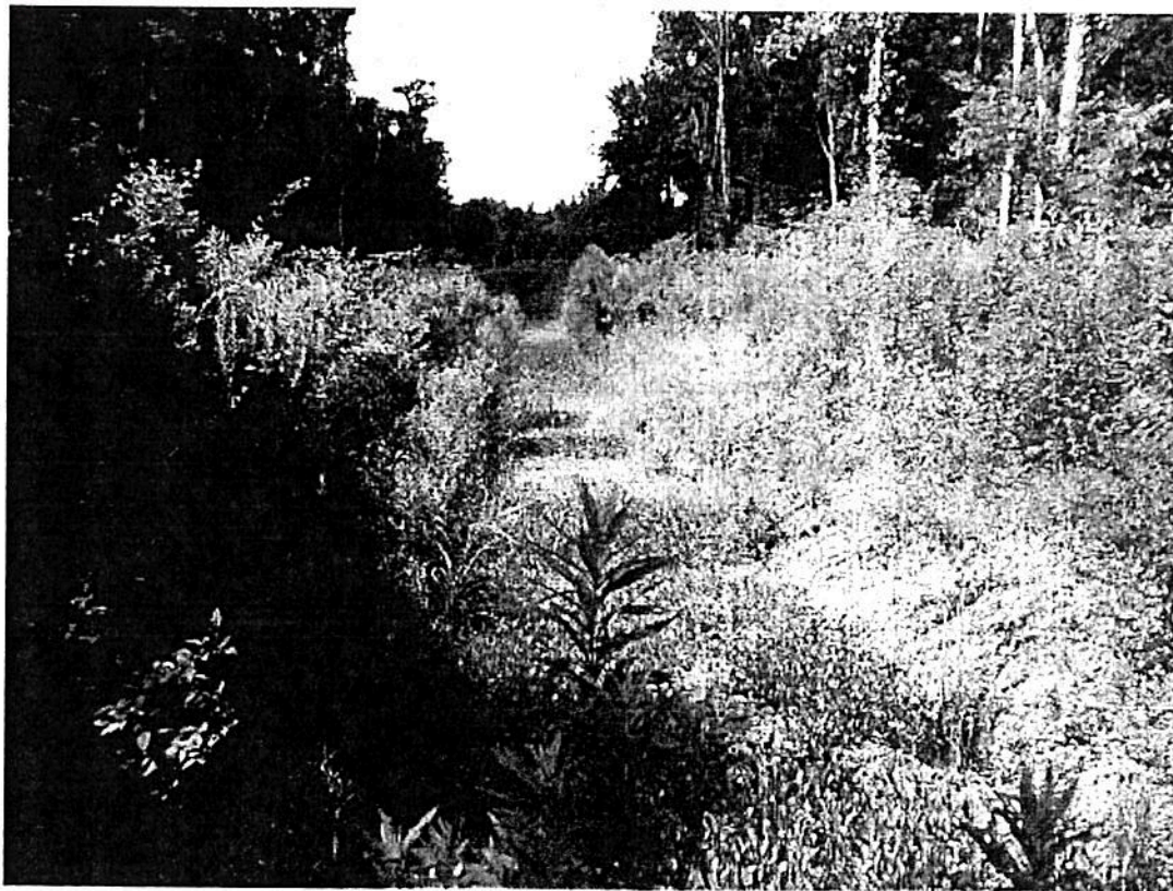
Photo #12 @ 7300' south of LA 1, viewing south towards the Forty Arpent Canal The cease and desist location of ditch being constructed 700' north of Forty Arpent Canal
