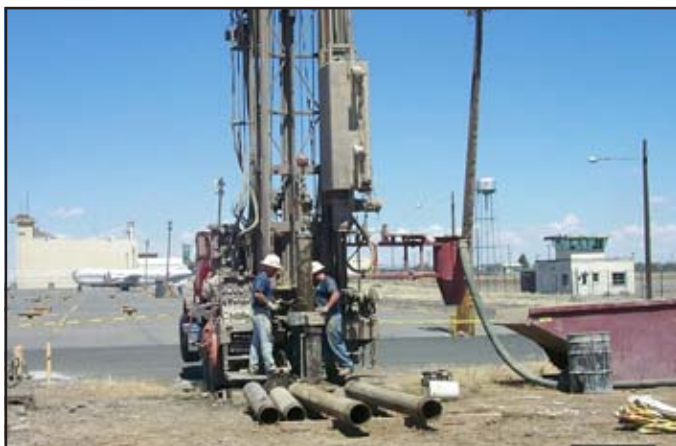
Drillers installed monitoring wells, which are tested periodically for groundwater contamination. (Montgomery Watson Harza photo)
