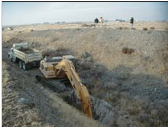
Workers dug trenches to search for contamination sources in landfills. (USACE photo)
